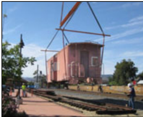
Caboose 409 is suspended in mid-air while it waits for its new trucks to be installed.
