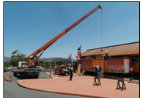
On Friday, July 19th, with help from Superior Crane , a gang of Museum volunteers saw cut around the perimeter of the floor, lifted the roof and walls and installed 14" crib walls. This was necessary to satisfy City Code for ceiling height in the restrooms.
