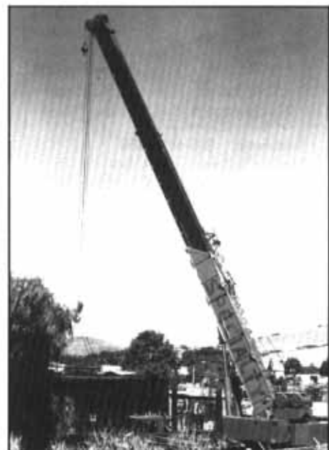
Specialty Crane of Santa Maria gently lifts boxcar from flatbed truck and . . .
